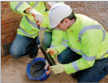
4. Check the piston is a snug fit in the cartridge and adjust in accordance with the pointing gun instructions. Load the mixture into the cartridge in the pointing gun immediately after agitating
